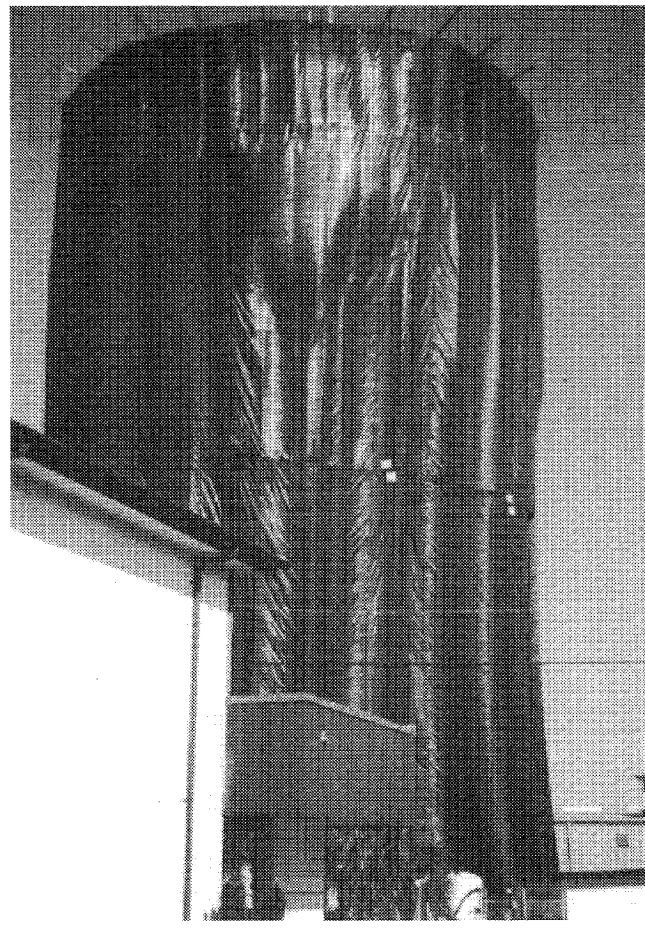
Total containment of an elevated water tank.
