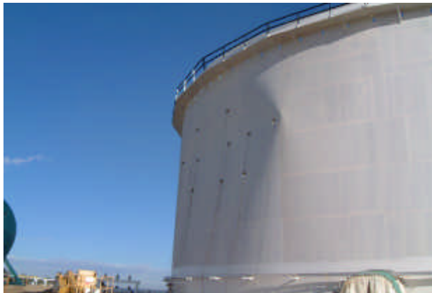
Tank Damaged by Wind (Before Pulling Out Dents)
