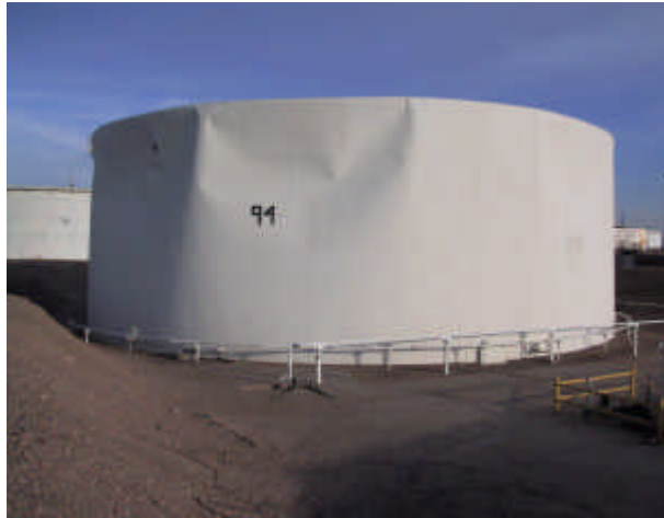
Tank Damaged by Negative Internal Pressure (Vacuum)
