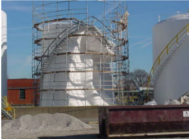
Tank Damaged Beyond Repair by Vacuum
