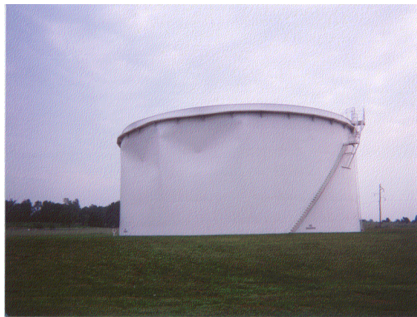
Tank Damaged by Tornado Winds
